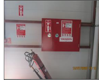
Photo of fire safety equipment Fire hose.JPG
