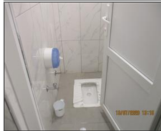
Photo of the sanitary facilities Lavatory.JPG
