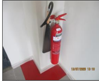
Photo of fire safety equipment Fire extinguisher.JPG
