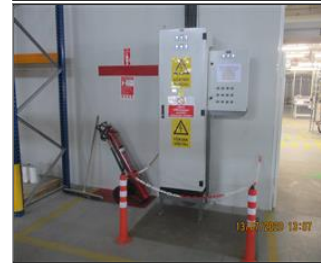
Photo of the inside of the main production hall Electrical control pannel.JPG
