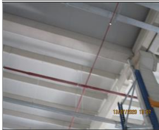
Photo of fire safety equipment Fire sprinkler system .JPG
